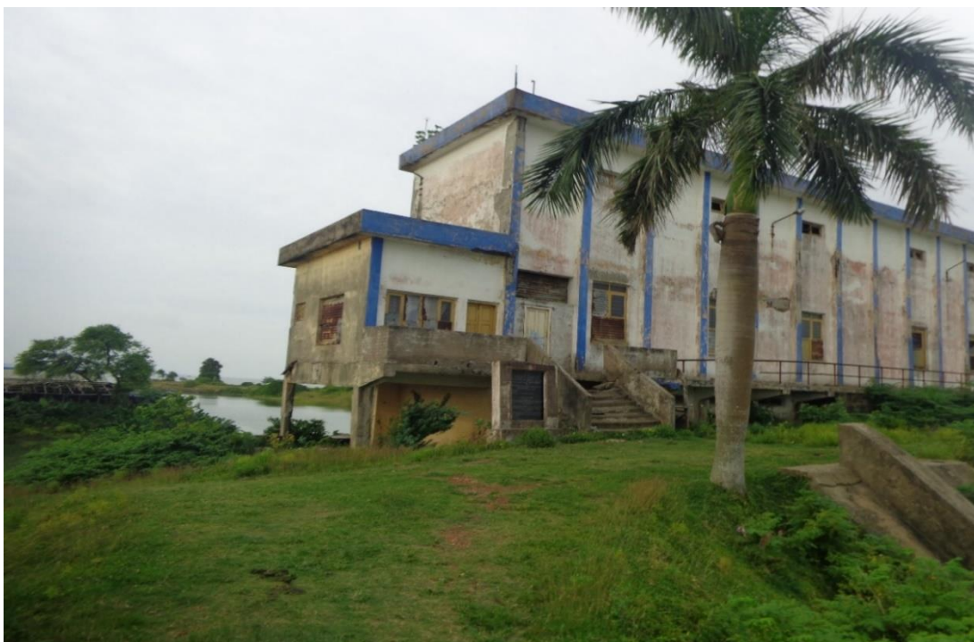
Image 111 : Defunct Building Of Fisheries Department On Nayachar Island [Purba Medinipur District]
